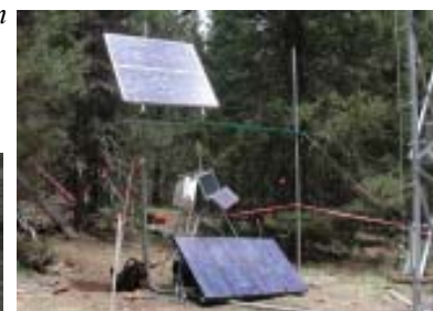
Power set up at the Spruce Site.
