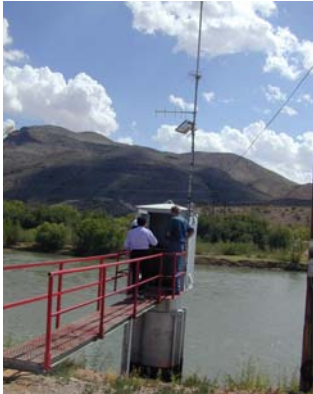
Telemetry Gage Station
